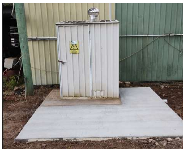
Photo from B Barwick: Work progressing at the Booral Site, the formwork and the new concrete slab which will form the floor of a larger shed in the future.
